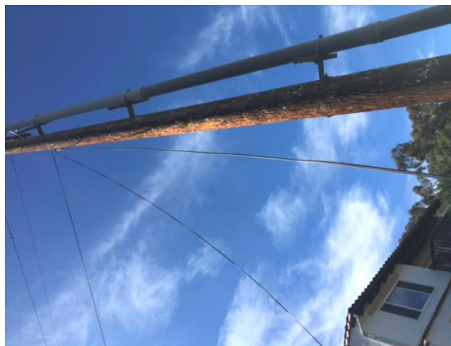
Telecommunication lines downed by speeder
